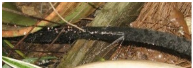
Rupture from high water pressure.
